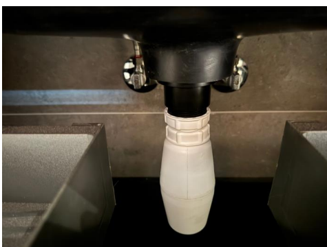
Røropplegg under servant.
